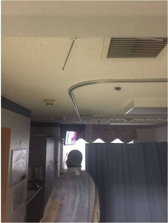
Photo 7 Supply diffuser in room 118 – staff is shown in photo
