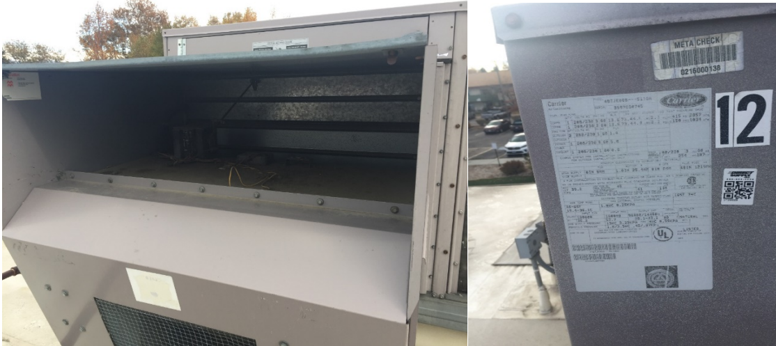
Photo 1 HVAC unit feeding rooms 120 and 118, note closed outside air intake lowers
