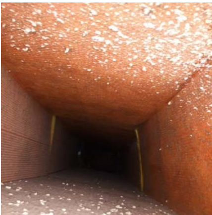
Photo 3 Inside of return air duct in room 120 - note insulation on the duct interior
