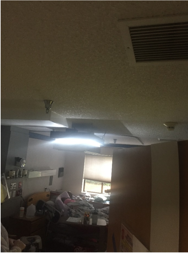
Photo 8 Halo unit suspended in room 120 with return air vent in the foreground – the supply diffuser can be seen on the ceiling past the smoke alarm
