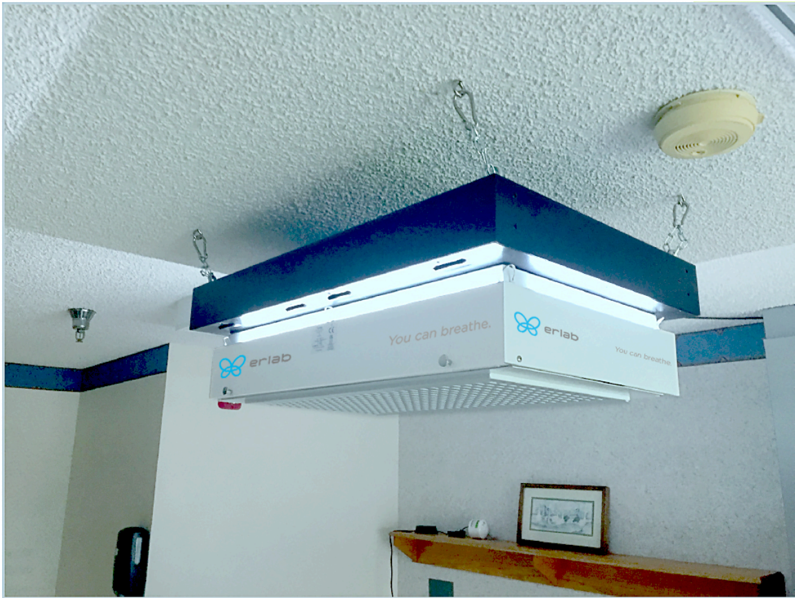
Photo 4 Ceiling mounted Halo HEPA filtration unit in room 120
