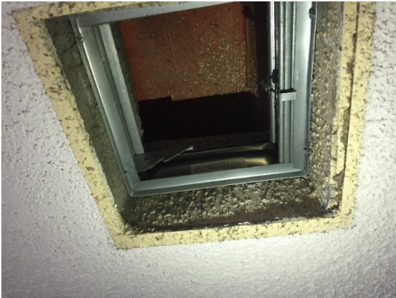
Photo 2 Return air vent in room 120- grill removed
